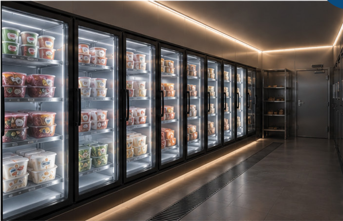
Cold Storage Facilities
